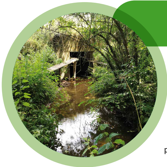
Adapting existing under-road corridors to make them attractive to local animals while monitoring them with cameras to assess their benefit. Marc Barra, ARB Ile-de-France.
